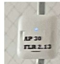
Close up of AP Box
